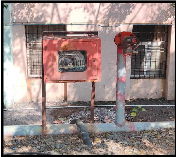
FIRE FIGHTING SYSTEM
